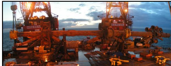
Severed Jacket Leg Onboard Crane Barge
