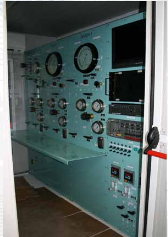
Picture 4. Control Room in Container
